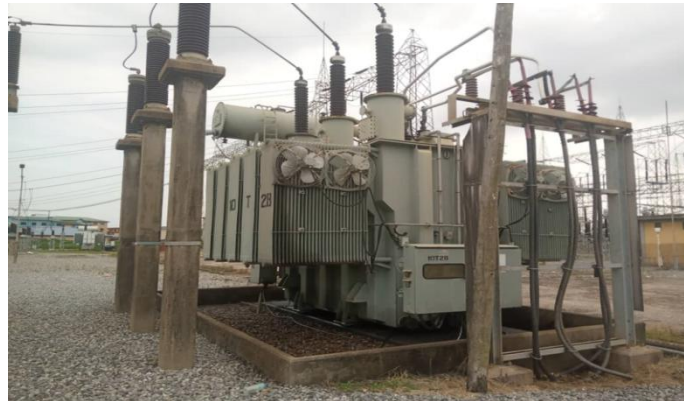
Figure 2: Akangba transmission substation (ats) power transformer
